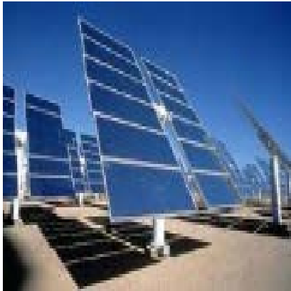
Solar electric panel
